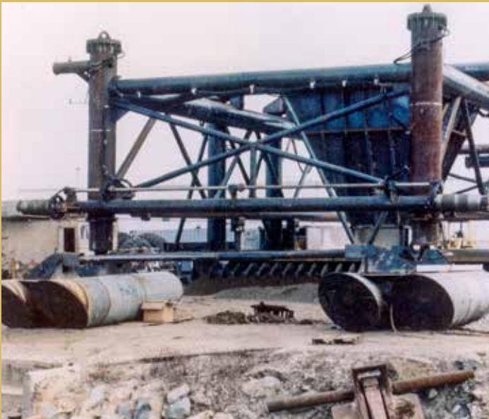
The screed was developed by the Joint Venture team to place the rock and sand “roadway” underwater to support the pipeline. PHOTO CREDIT | POINT LOMA OUTFALL PROJECT TEAM
