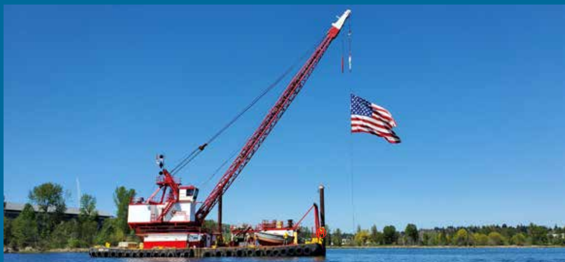
Manson's derrick barge DERRICK 6 in Lake Washington near the University of Washington's Husky Stadium. PHOTO CREDIT | DREW EDWARDS—HEAVY LIFT AND MARINE SUPERINTENDENT
