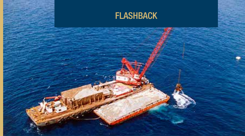
The derrick barge HAAKON placing rock on the Point Loma Extension project, San Diego, CA. PHOTO CREDIT | HAWKINS PRODUCTIONS
