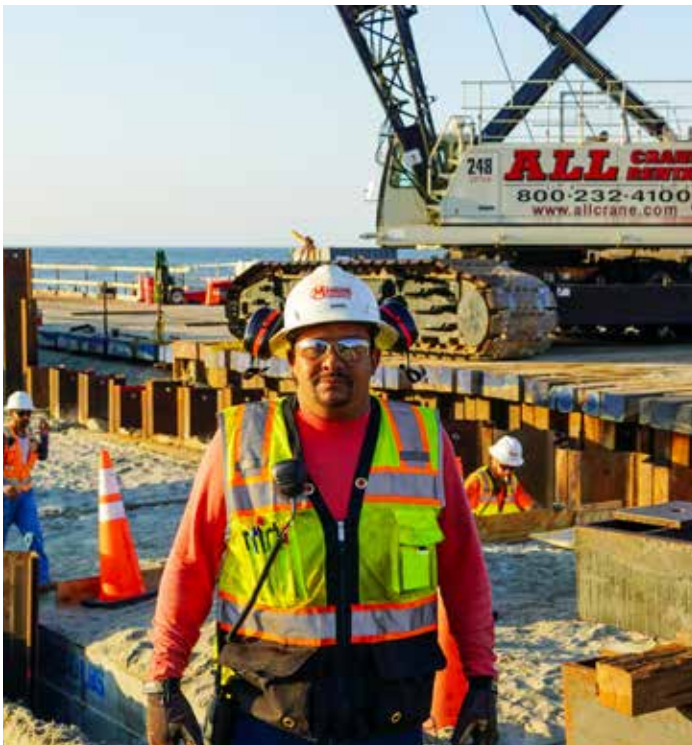
Piledriver Foreman Miguel Delgado just after his morning meeting with the piledriving crew at 18th Ave North.
