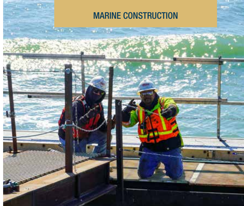
Two members from the piledriving crew take a second to pose on the trestle walkway. (L-R) Piledriver Fermin Chavez Lugo and Piledriver Foreman Miguel Delgado.
