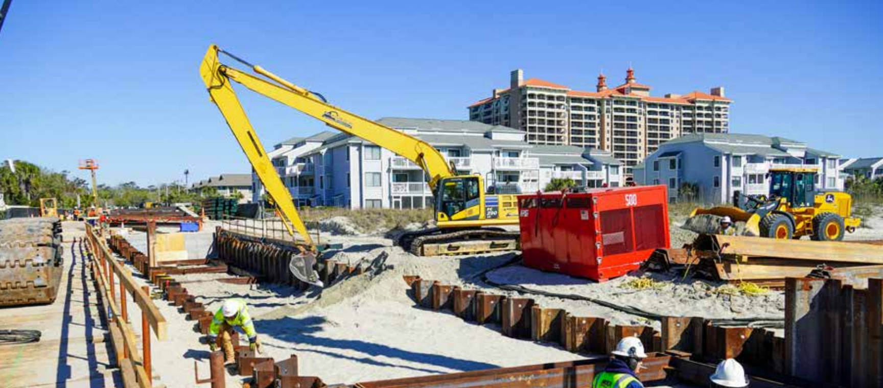
A view from the trestle of the 18th Ave. North Ocean Outfall crew working safely to remove material from the cofferdam. PHOTO CREDIT | J. ANTHONY TEDPAHOGO—COPYWRITER
