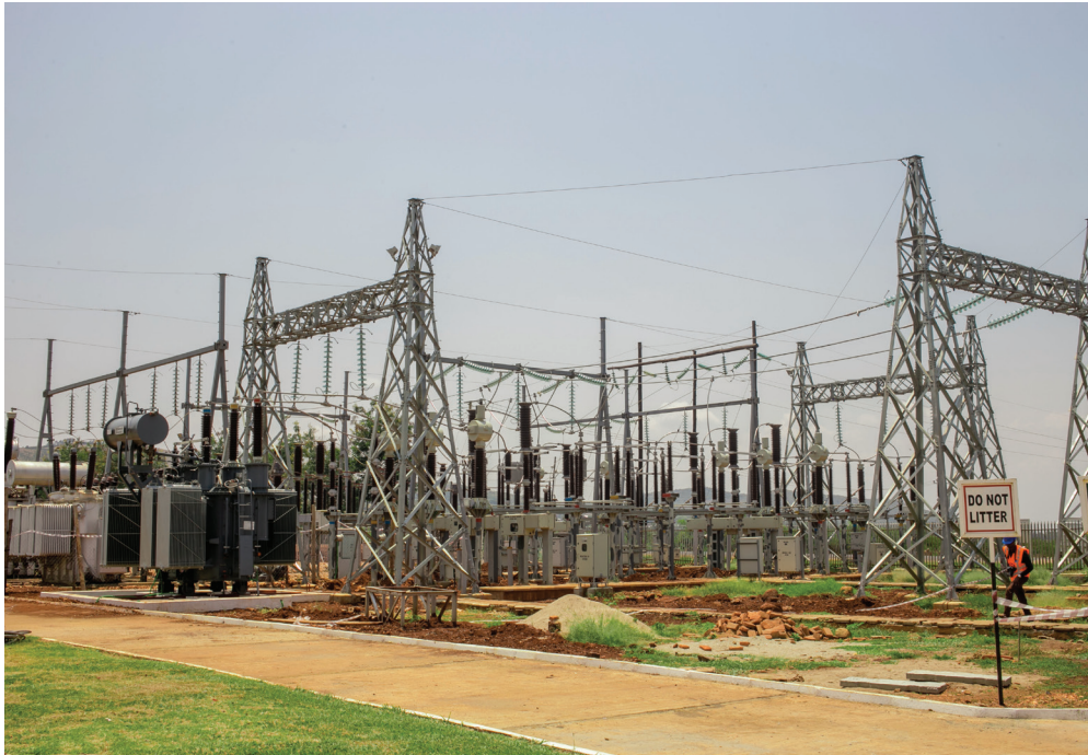
The UETCL Nkenda Substation is a key component for adequate power evacuation of GET FiT hydropower projects in Western Uganda. Photo: GET FiT
