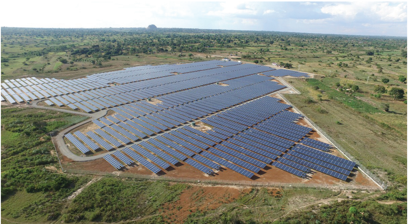
Soroti Solar Power Plant. (photo: Access Power)
